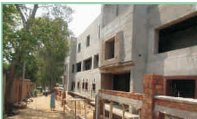
Construction of GPL Standard Invivo Laboratory at Indian Institute of Integrative Medicine (IIM), Jammu
